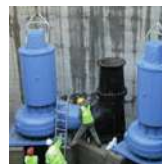
IRELAND Maintaining pressure at pumping stations
