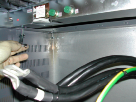
Inverter and FSU connection together
